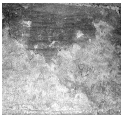
Fig. 3. The concentration of soluble salts present on the wall subsurface; as sub-efflorescence.
