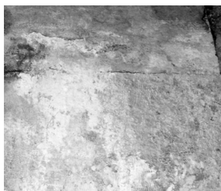
Fig. 2. The concentration of soluble salts present on the wall surface; as efflorescence.
