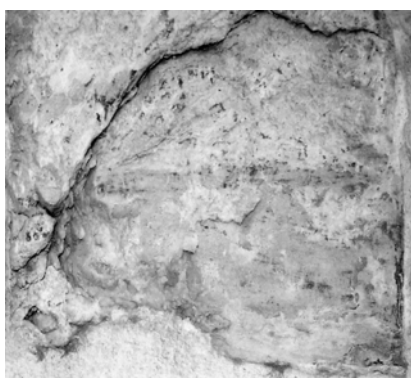
Fig. 1. Scales, one of the common superficial detachment forms.
