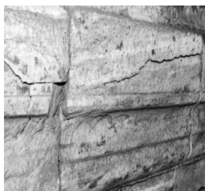
Fig. 4. Cracks extend in an irregular way close to the horizontal.
